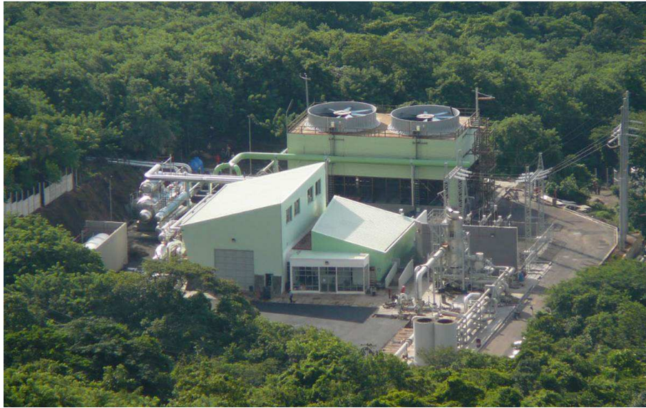
Figure 24 : Photography of the power plant from Berlin to Salvador equipped with a combined cycle powered by 109 MWe (© Verkis).
