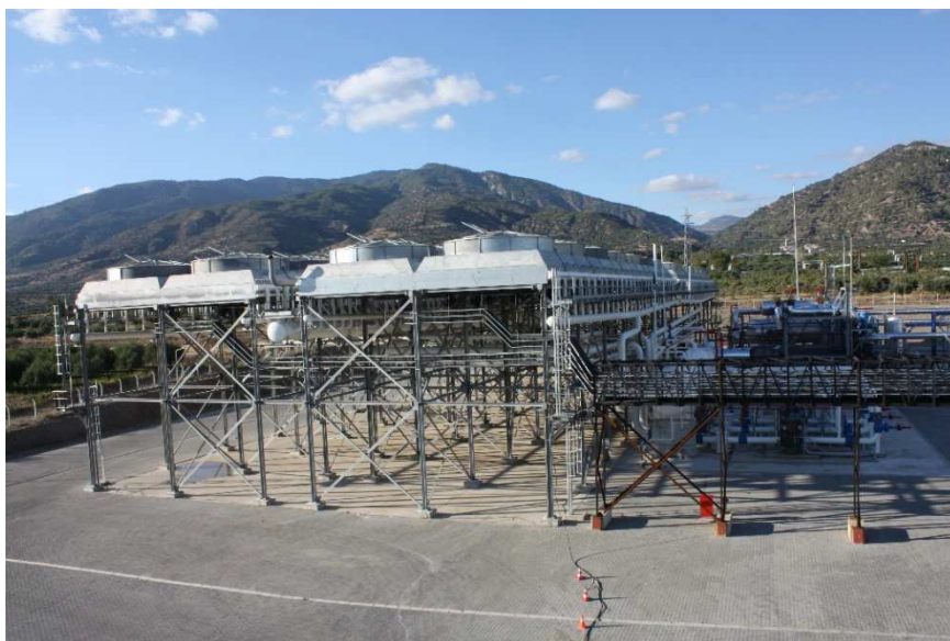
Figure 4: Cooling air system in the power station of Pamukören in Turkey. (ORC type turbine 2x25 MWe of Design Atlas Copco Energas ; ©Verkis).
