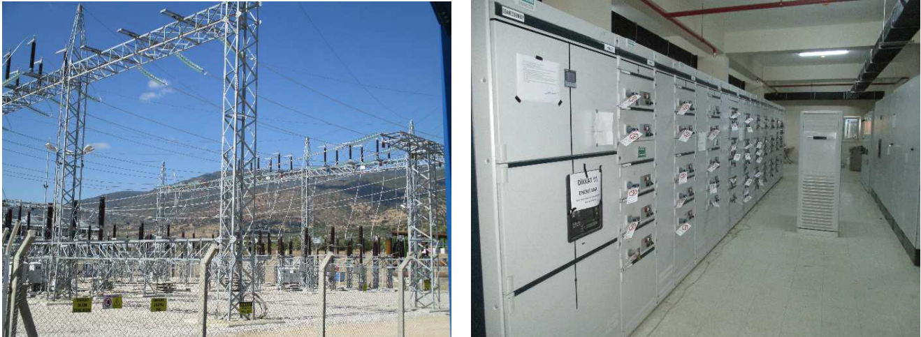
Figure 17 : Picture of an electric substation and a room for electrical equipment in the power plant of Pamukören in Turkey (© Verkis).
