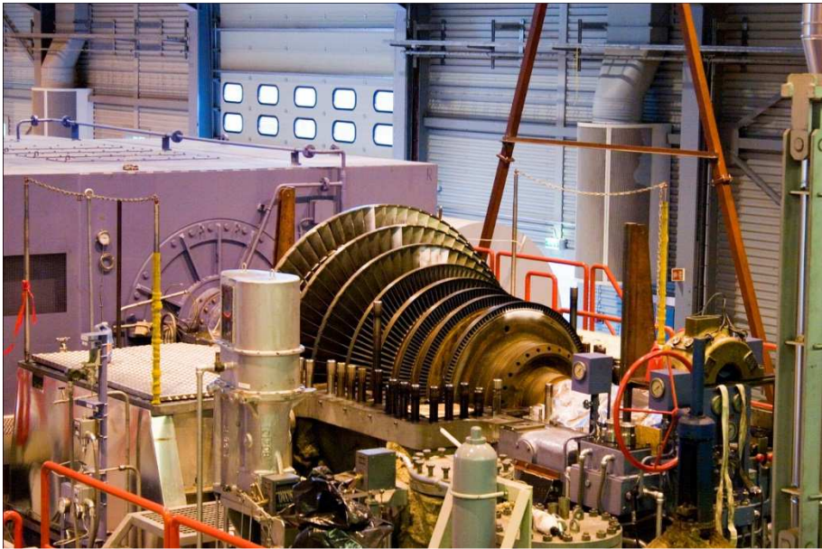
Figure 15 : Picture of the rotor of one of the steam turbines in the power plant of Hellisheidi in Iceland during its construction (© Verkis).
