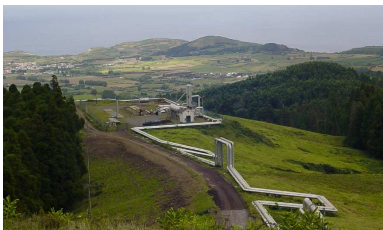
Figure 13 : System of transport of the fluids to the power plant of Pico Vermelho in the Azores (© CFG Services).
