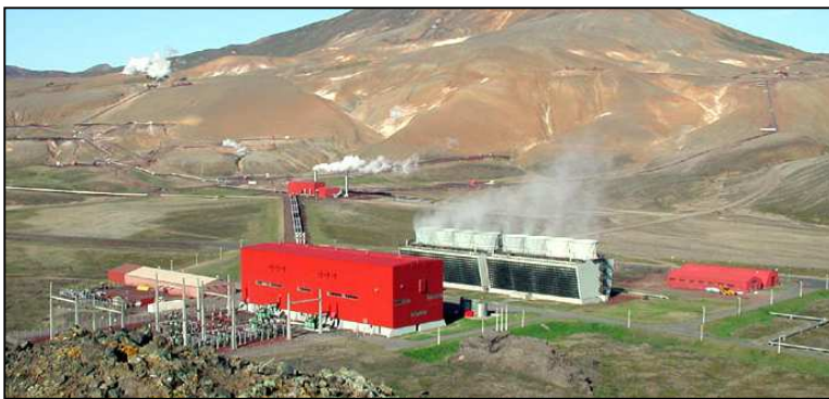
Figure 16 : Cooling towers on the geothermal power plant of Krafla in Iceland with a capacity of 60 MWe (© Verkis).
