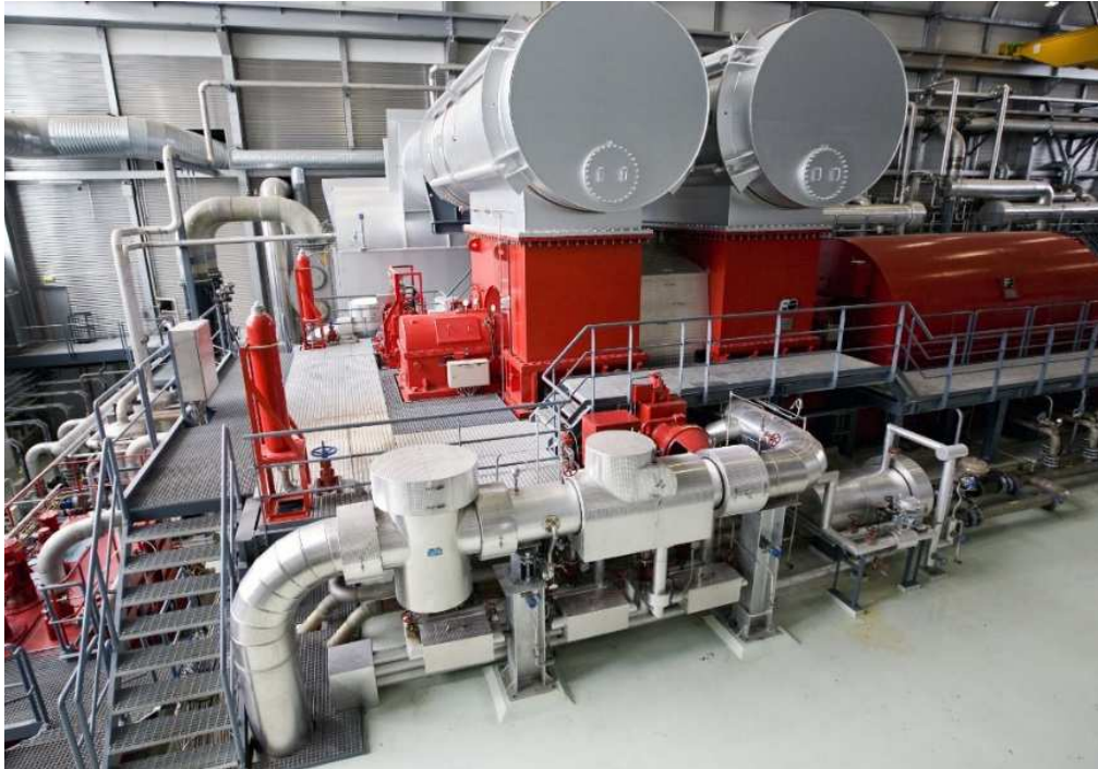
Figure 14 : Picture of a Fuji steam turbine with a capacity of 50 MWe in the geothermal power plant of Reykjanes in Iceland (© Verkis).
