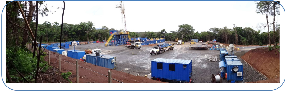
Figure 22: Organisation of a development drilling site, in the lands of Las Pailas, Costa Rica, made by ICE (©Biotope).
