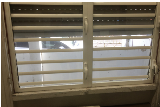
FIGURE 19. Example of an airtight blind. In the closed position, the slats are tightened on a horizontal riser provided with an elastomer seal that provides airtightness..
