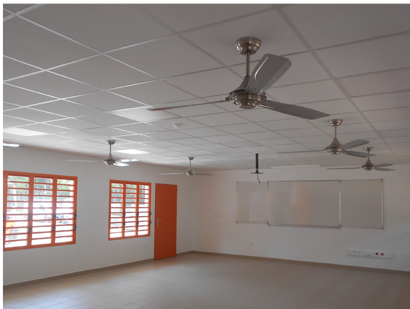
FIGURE 15. Example of premises equipped with ceiling fans.
